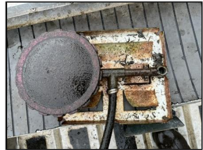
Figure 12: One of two broken aeration diffusers within Hills Pond
