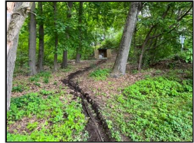
Figure 4: A trench was created from the power box to the shoreline of the Pond for the aeration hosing
